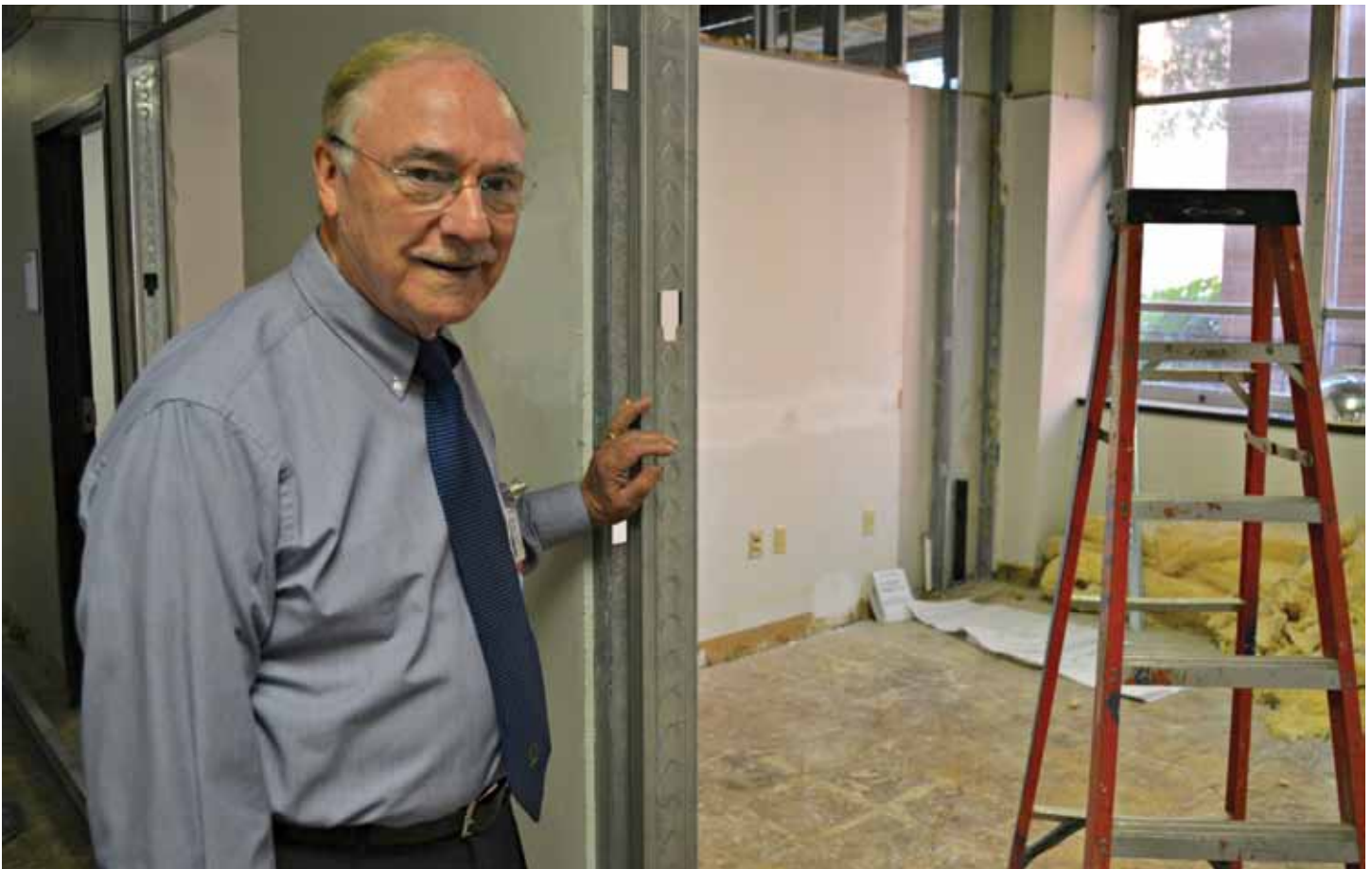
Charles Cranford, D.D.S., director for the Center for Dental Education, looks over construction at the future oral health clinic, set to begin accepting patients in January 2013. The clinic is being created from renovated space adjacent to the existing dental hygiene clinic.
